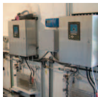
Field remote terminal.
