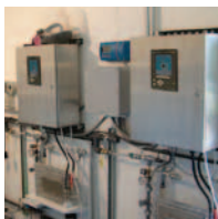
Field remote terminal.
