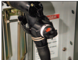
A Test Point Reset Fault Indicator with junction shield provides indication in a switchgear cabinet.
