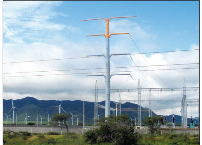
First substation energized with true multisupplier integrated system using IEC 61850—La Venta II substation, Juchitán, Oaxaca, Mexico.
