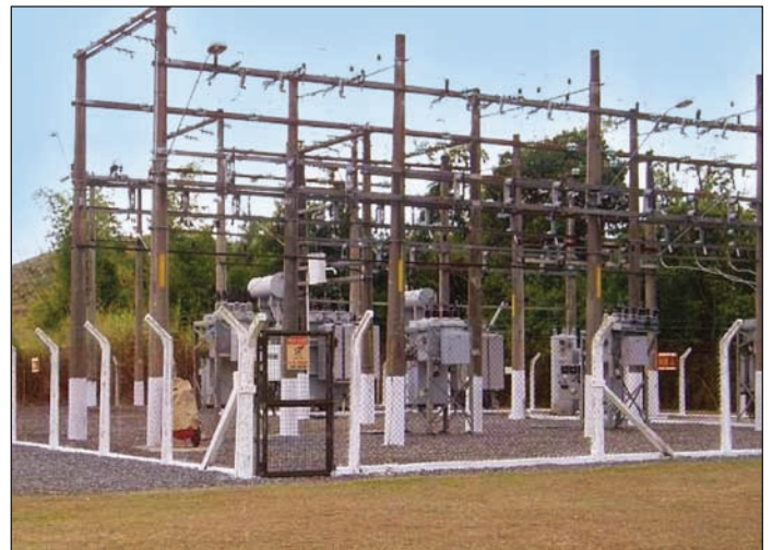
Guarujá 2, the first of 30 substations energized in a major modernization project for Elektro Eletricidade e Serviços in Brazil.
