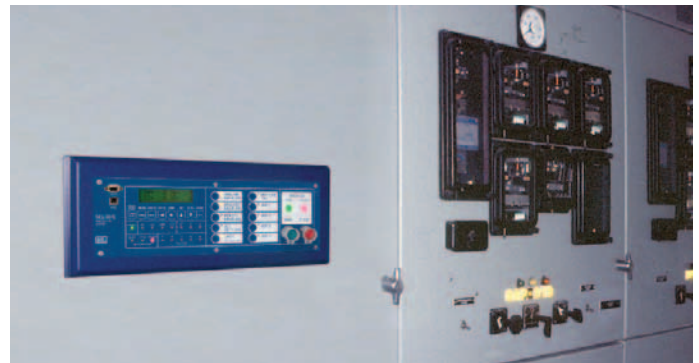
One SEL-351S Protection System replaced an entire panel of EM relays.
