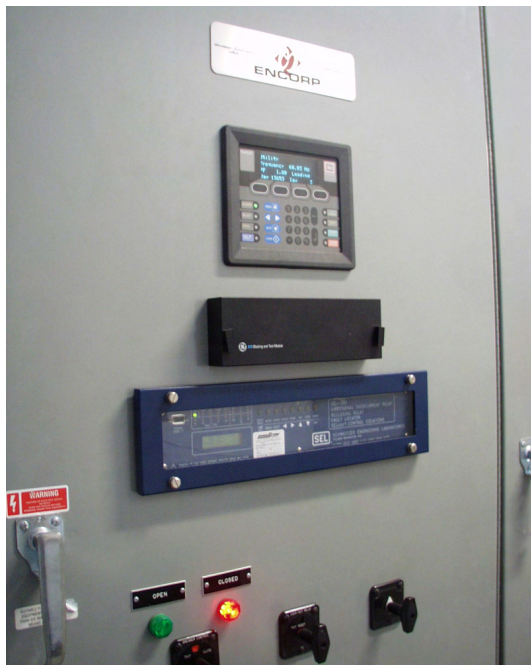
Figure 2—Encorp selected the SEL-351 Directional Overcurrent and Reclosing Relay (shown above) to provide interconnection protection.
