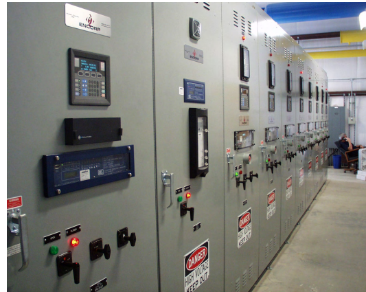
Figure 1—After preliminary evaluations, both CNP and NOBEL/SYSCO incorporated solutions provided by Encorp based on natural gas genset power sources and Schweitzer Engineering Laboratories, Inc. (SEL) microprocessor-based relays for monitoring, control, and protection.
