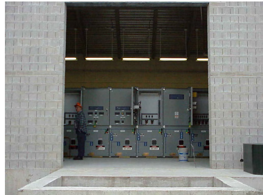
Figure 1—In response to 1998 Energy Competition Act, Barrie Hydro had the opportunity and challenge to provide reliable, high-quality electricity and customer services. This led to a project to improve the protection, data collection, and automation of the distribution system that began in 2000. Shown above is one of the four new substations built to provide important communications and automation capabilities.
