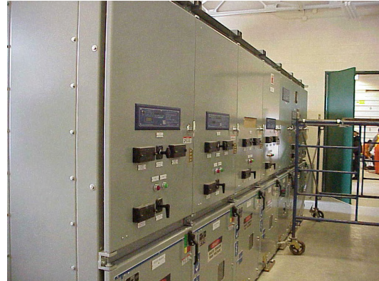
Figure 2—“We had successfully used arc-proof, metal-clad switchgear with, typically, a four-feeder substation... We decided to use microprocessor-based relays, which our investigations showed were highly reliable and could provide important communications and automation capabilities,” explains Doug Fairchild, Planning Engineer at Barrie Hydro.
