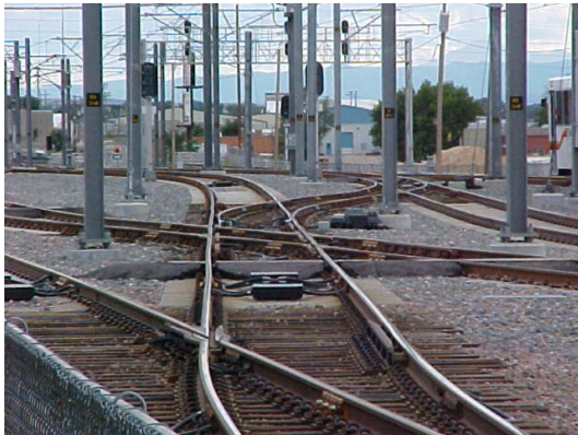
Figure 2—Shown is the Denver RTD light rail switching tracks at the Broadway Station. The Denver LRT system will have a total of 120 miles of track once the project is complete in 2016.
