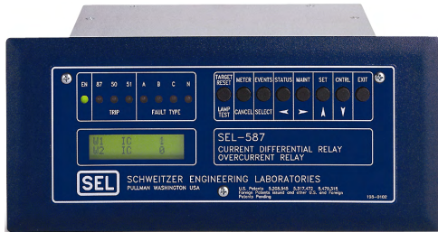
Figure 2—For monitoring and protection, MCI used the SEL-587 Current Differential Relay, which provides oscillographic event reports and metering functions that reduce or eliminate external recorder and metering requirements.
