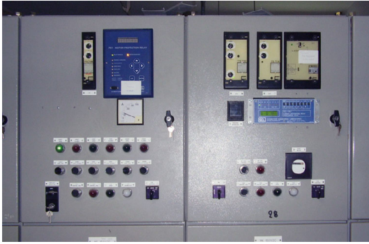
Figure 4—For an economical, high-speed retrofit, MOH abandoned the existing protection and metering, and installed new SEL relays in the switchgear.
