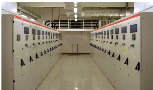
Figure 3—MOH directed switchgear manufacturers to purchase and install SEL protective relays in new installations.
