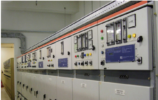
Figure 5—SEL relays protect all MOH's major electrical system assets.
