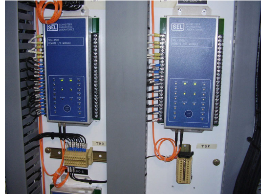
Figure 6—Ultrahigh-speed, remote-mounted I/O modules were installed throughout the plant for the SEL POWERMAX load-shedding system. These control (DIP) switch-configured I/O modules have trip-rated output contacts, devoted communications, on-board power supplies, and full self-monitoring for the utmost reliability.
