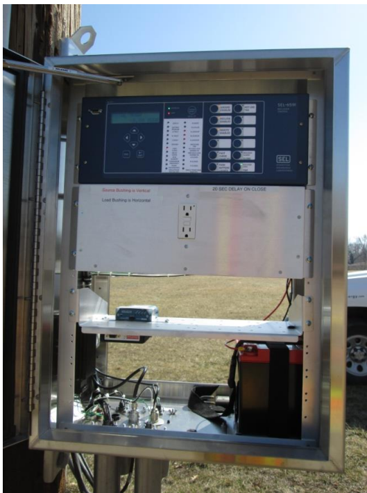
Figure 2—SEL-651R Advanced Recloser Control, SEL-2401 Satellite-Synchronized Clock, and 3G Cellular Modem
