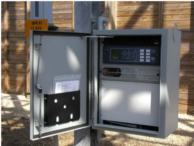
Fig. 7. A smart, automated, and distributed device installed local to the grid apparatus that it protects, controls, and manages
