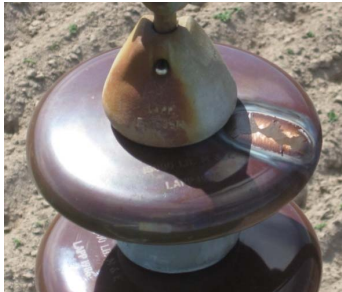
Fig. 14. Damaged insulator at 98.98 kilometers from the Goshen terminal.
