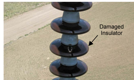
Fig. 11. Damaged insulator at 109.29 kilometers from the Goshen terminal.
